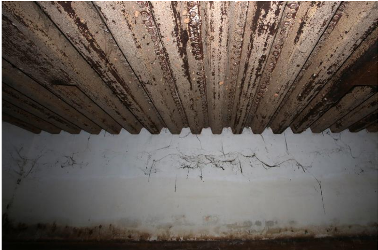
Fig 2. The inclined corrugated ceiling of the building structure where the bat was found roosting.
