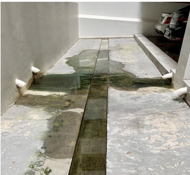
Fig 1. Drain on the ground floor of a multi-storey carpark where the clouded assimininid snails were found. (Photograph by: Lau Wing Lup).
